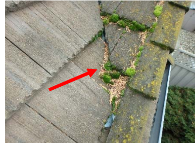
Example – Debris in Valley
