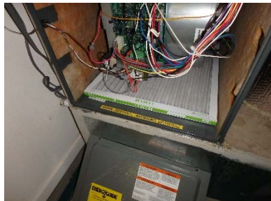
Air Filter Inside Furnace Cabinet
