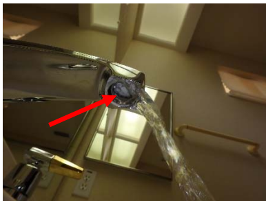
Example – Missing Aerator
