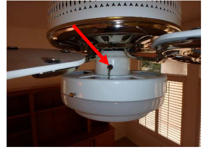
Fan Speed Control – Family Room
