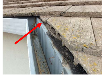
Deteriorated Roofing Paper
