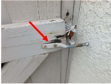
Example – Loose gate Latch Arm
