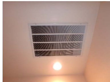
Return Air Grill in Hallway
