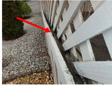
Example – Loose Fencing Slats
