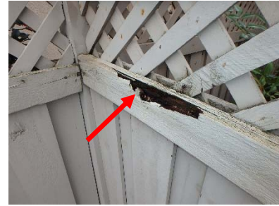
Example – Deteriorated Fencing
