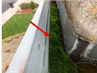
Example – Debris in Gutter
